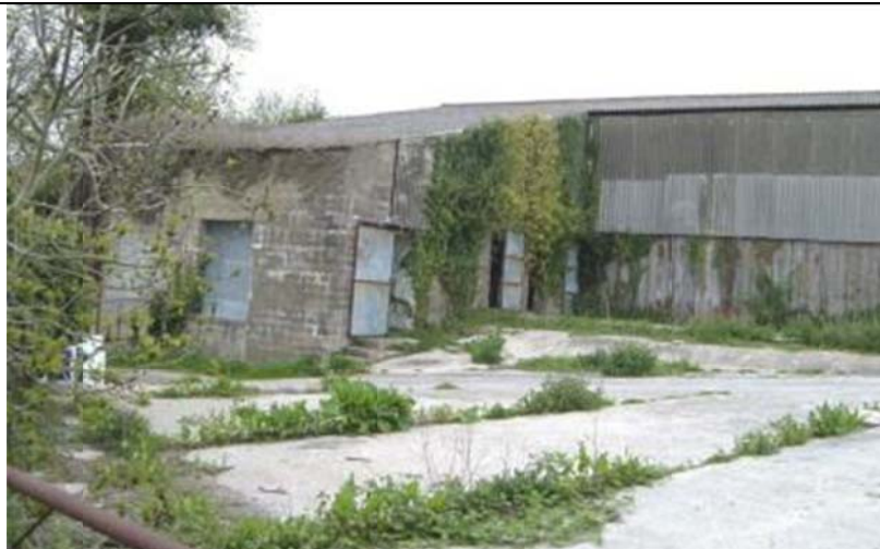
Figure 3-1: A picture showing a derelict space in Blandford St. Mary village, district of Dorset, England.
